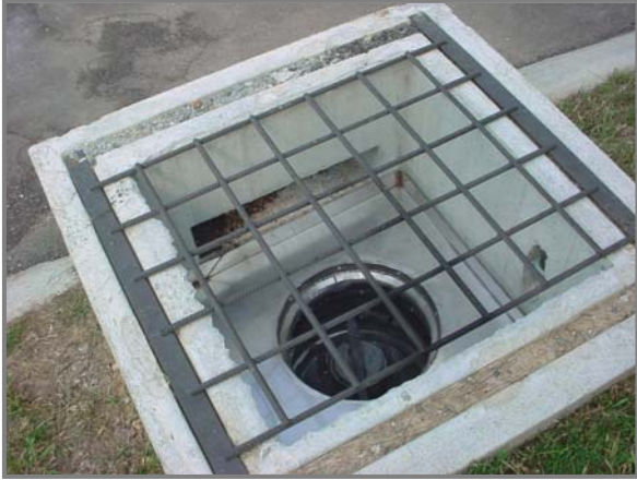
The surface grate over an Aqua-Guardian™ unit
